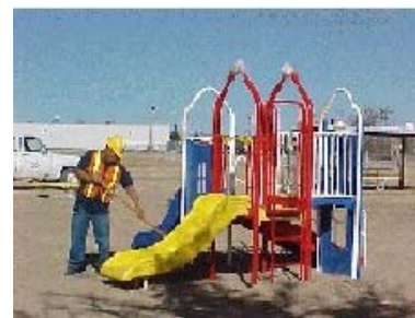
Mario Hernandez removing rocks from the sand around the new playground equipment.
